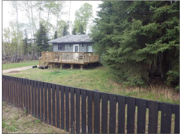
Combustible Un-Skirted Decking
